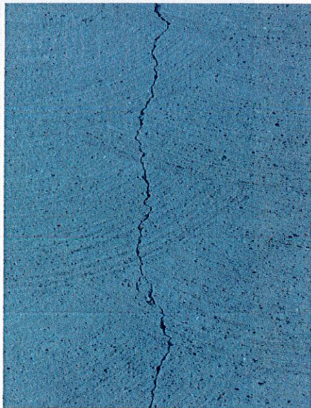
Figure 2. An example of a restraint crack. Cracks typically extend through the depth of the member.
