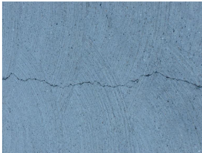
FIGURE 1-2 Example of a Restraint Crack (P751) Restraint cracks are generally long, wide, extend through the depth of the member and occur at axially weak locations, such as where the reinforcement ends.
