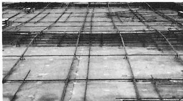
View of a two-way flat slab in the direction of distributed tendons prior to placement of concrete.
