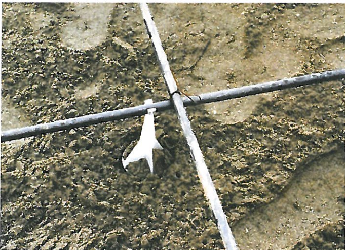
Fig. C.11-1—Close view of a ground-supported slab in building construction ready to receive concrete.
