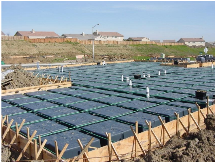
FIGURE 1-4 VIEW OF POST-TENSIONED WAFFLE FOUNDATION SLAB Post-tensioned waffle slabs are also used for foundations of low residential buildings, where seasonal volumetric changes in the foundation soil result in unacceptable soil movement at the structure's perimeter
