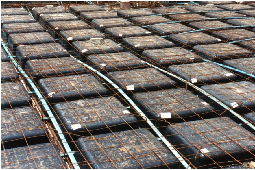
FIGURE 1-2 VIEW OF POST-TENSIONED WAFFLE SLAB CONSTRUCTION Interior span with PT tendons in each stem
