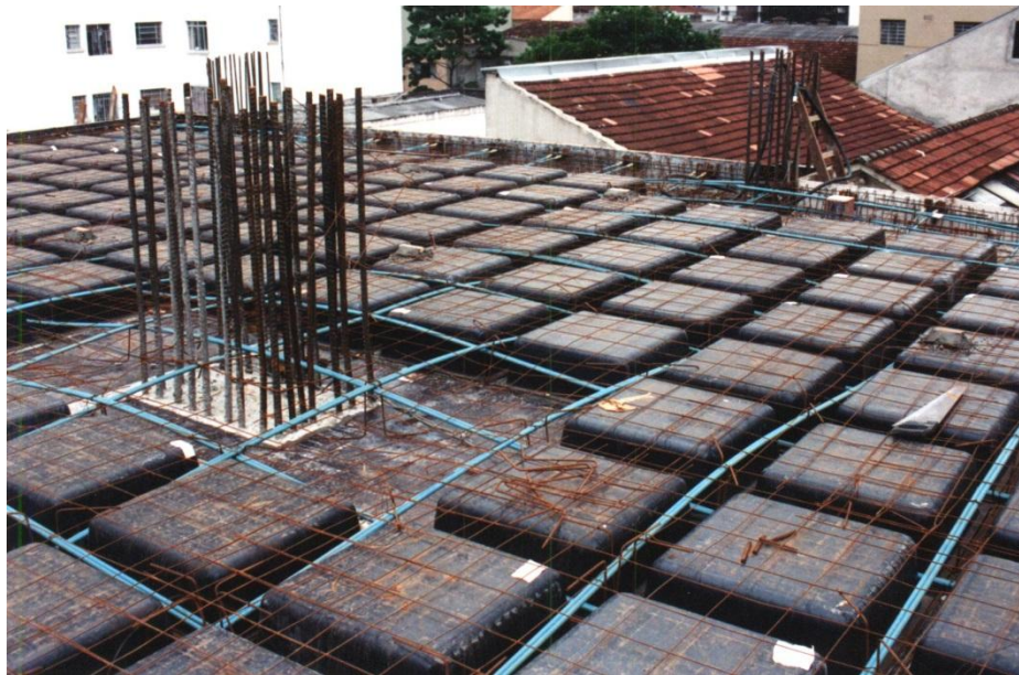
FIGURE 1-1 POST-TENSIONED WAFFLE SLAB CONSTRUCTION Each waffle stem is provided with post-tensioning tendons
