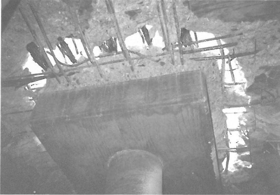
PICTURE 18: THE REBAR AND STRAND ACROSS THE OPENED GAP WERE FLAME CUT.
