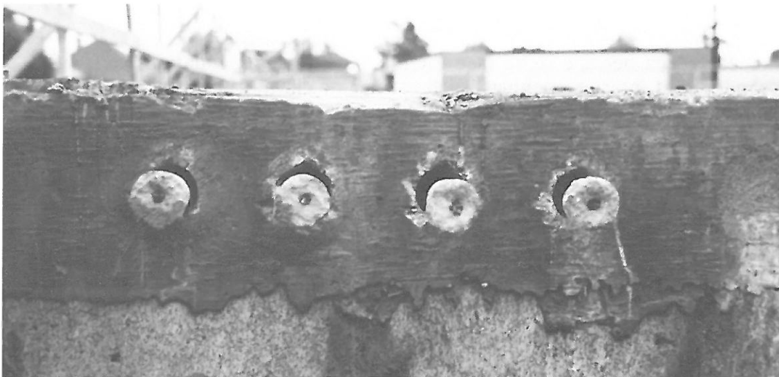
PICTURE 12: NOTE THE GROUT PLUG PUNCHED THROUGH BY THE KERN WIRE.
