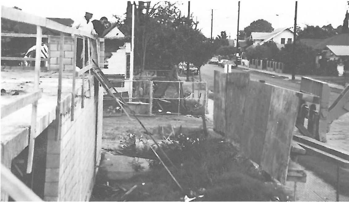
PICTURE 10: PLYWOOD SHIELD RAISED WITH A FORKLIFT TRUCK AND HELD IN LINE OF THE STRANDS BEING CUT.
