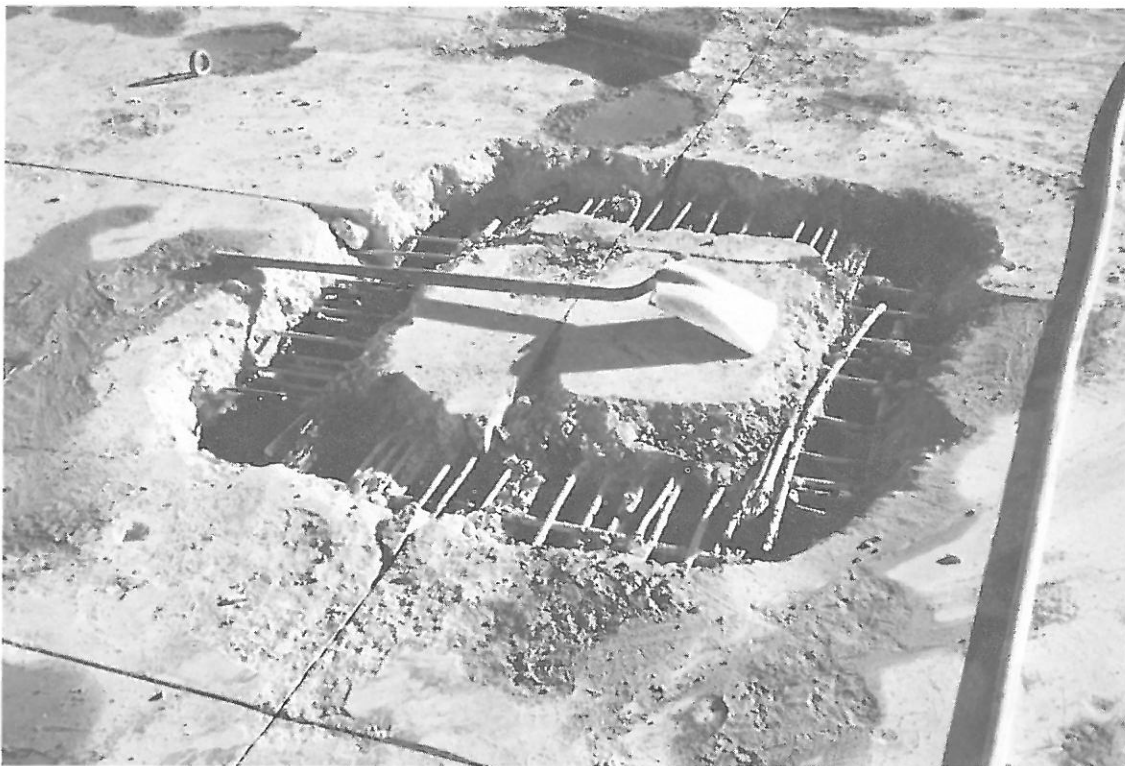
PICTURE 17: THE COLUMN CAPITALS WERE CLEARED FROM THE SLAB USING PNEUMATIC TOOLS.
