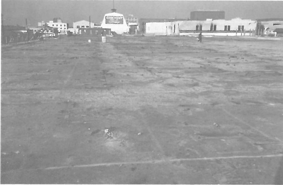
PICTURE 8: VIEW OF THE PODIUM SLAB AFTER CLEARING THE REMAINS OF THE BURNT WOOD FRAME AND MARKING THE SEGMENTS FOR DEMOLITION.
