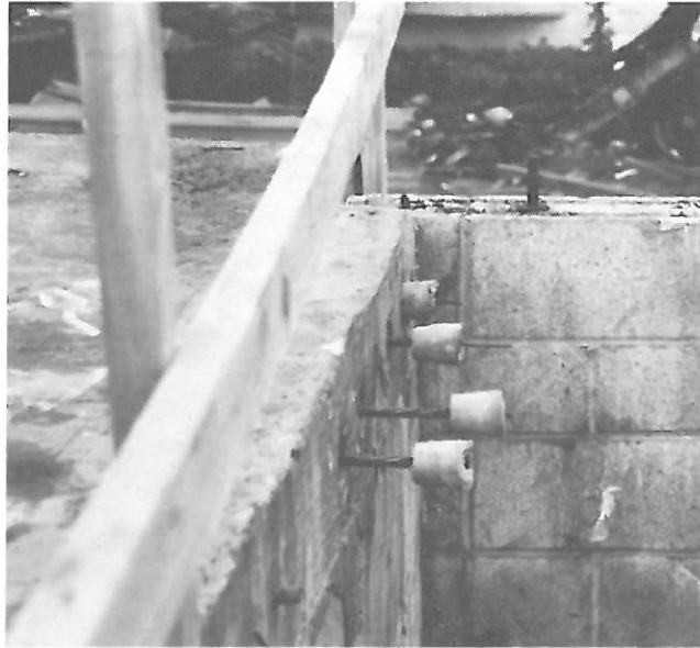
PICTURE 11: SLAB EDGE CONDITION AT LOCATIONS OF DISLODGED TENDONS.
