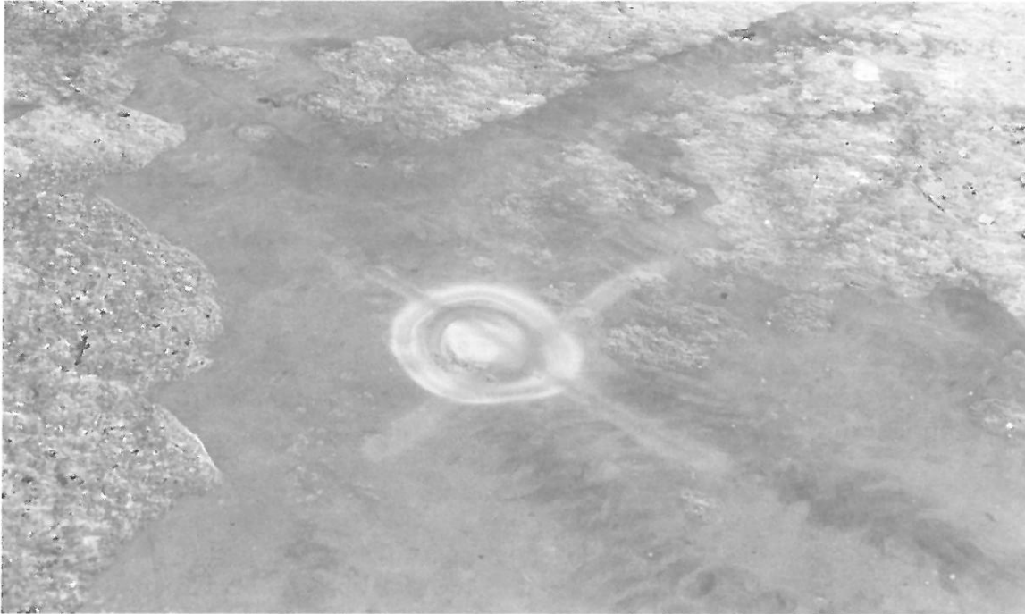
PICTURE 2: COLUMN LOCATIONS ARE MARKED ON SLAB SURFACE. CONCRETE DETERIORATION IS MINIMUM OVER COLUMN SUPPORTS.
