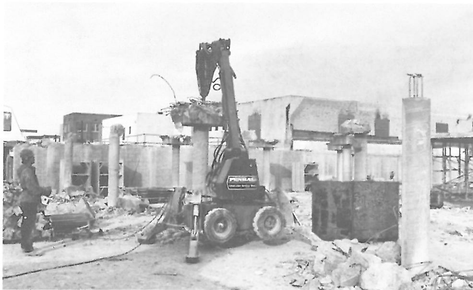
PICTURE 24: PNEUMATIC TOOLS WERE USED TO CHIP OFF THE COLUMN CAPS TO THE TOP OF THE COLUMN.
