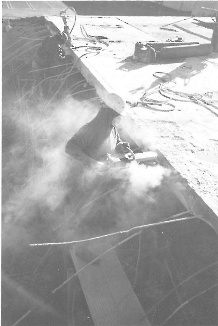
PICTURE 27: PREPARATION OF THE SLAB EDGE OF THE RETAINED SLAB PORTION FOR RECOVERY OF ITS POST-TENSIONING.
