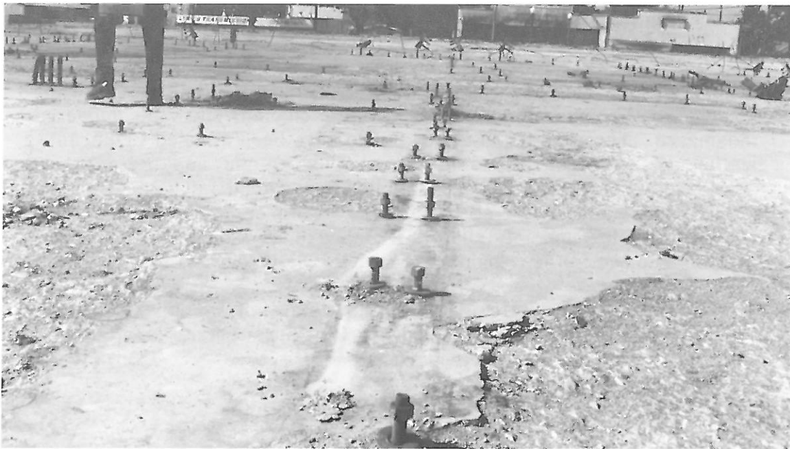
PICTURE 3: REMAINS OF ANCHOR BOLTS AT LINE SUPPORTS. OBSERVE CONCRETE SPALLING AWAY FROM THE SUPPORT LINE.
