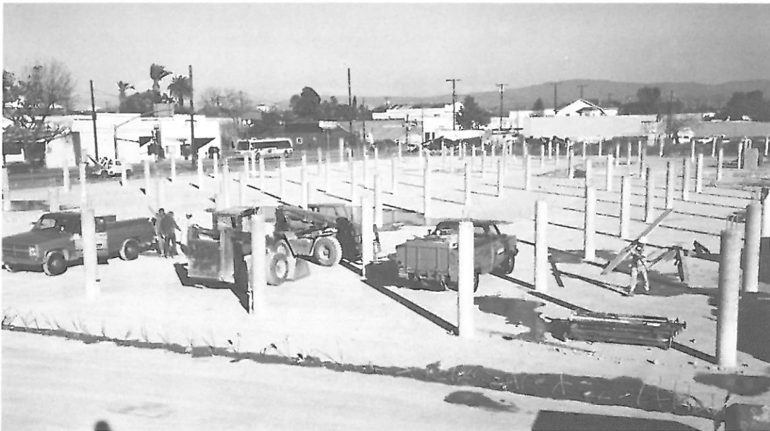
PICTURE 25: VIEW OF THE STRUCTURE AFTER COMPLETE REMOVAL OF THE UPPER POST-TENSIONED SLAB.
